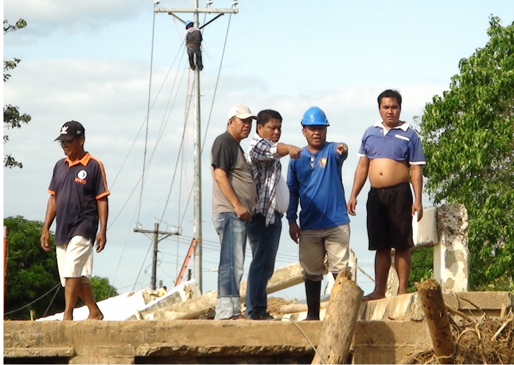
GM Oledan together with the Naval Water District general manager and the municipal engineer discussed how to reconstruct the damaged water pipe lines along the bridge of Caraycaray.
