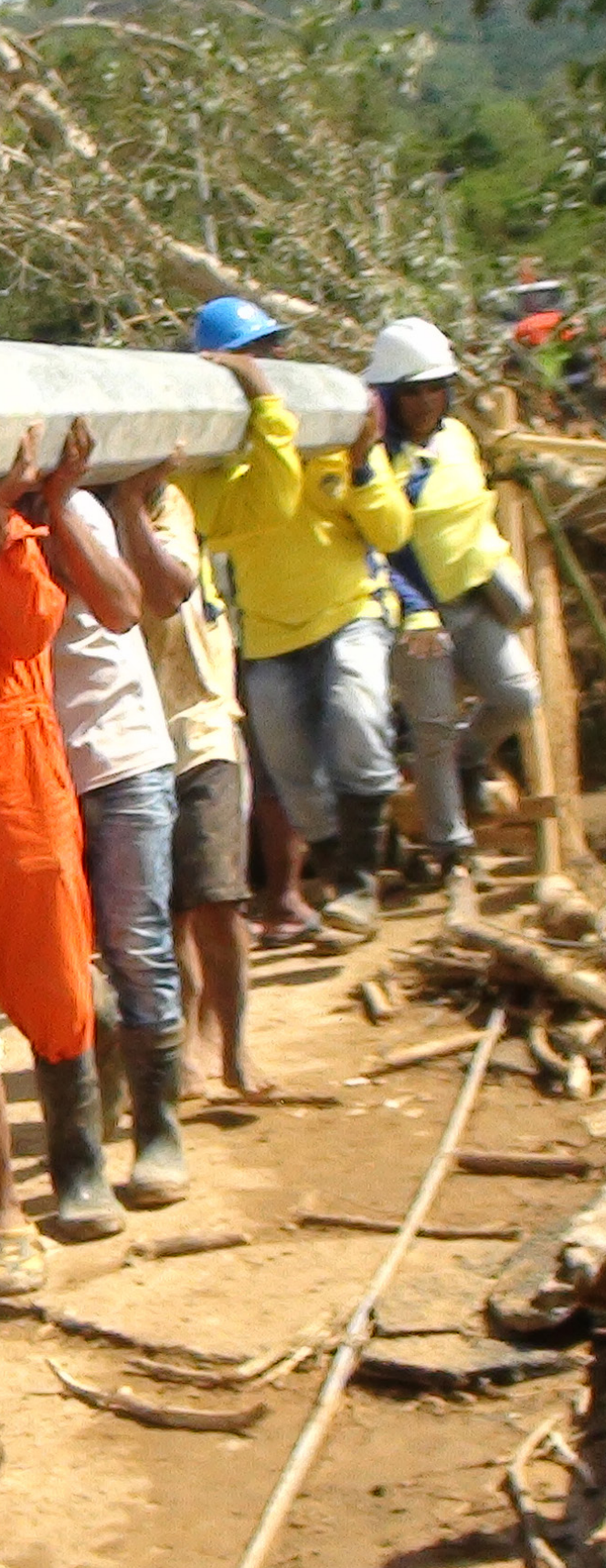
Linemen employed physical strength to carry this steel pole to the other end of the bridge.
