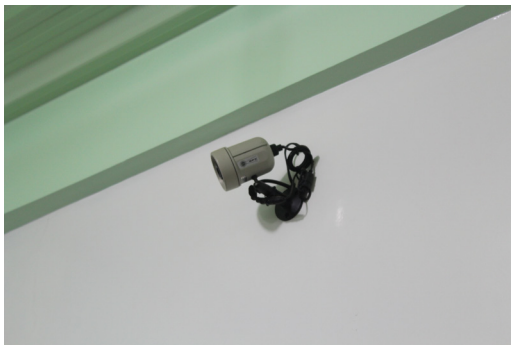
Installation of CCTV Cameras
